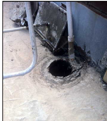
The downpipe in the middle of the gutter which brings the rainwater down to the Mikvah .
