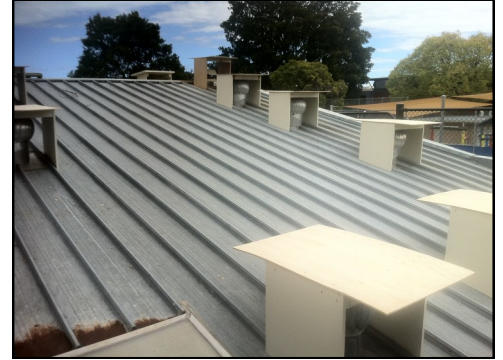
The flat sloping roof catches the rainfall. The roof is constructed with no exposed screw heads which could be considered receptacles.
