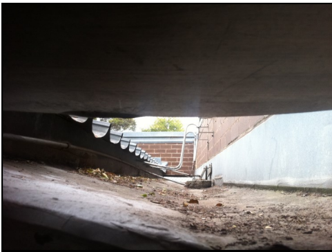
The gutter at the bottom of the roof is constructed with open sides so as not to be classified as a receptacle.
