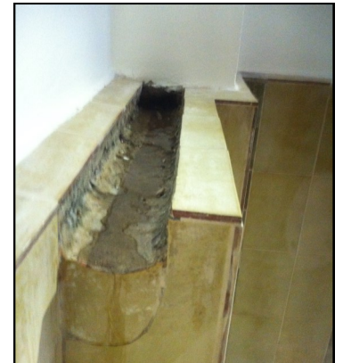
The water comes down the pipe and runs through the Hamshacha channel before entering the Mikvah .
