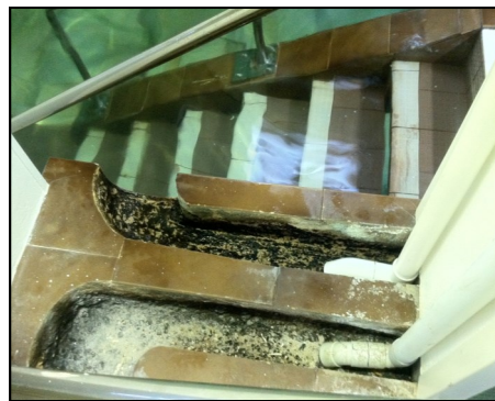
Once the rainwater is full, the tap water is brought into the upper Mikvah coming through a separate hamshacha channel.
