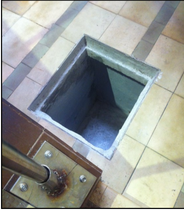
The Bor Tachton for containing the rainwater. Typically holds over 660L of rainwater. Note the ledge on which the stone cover will be placed once filled.
